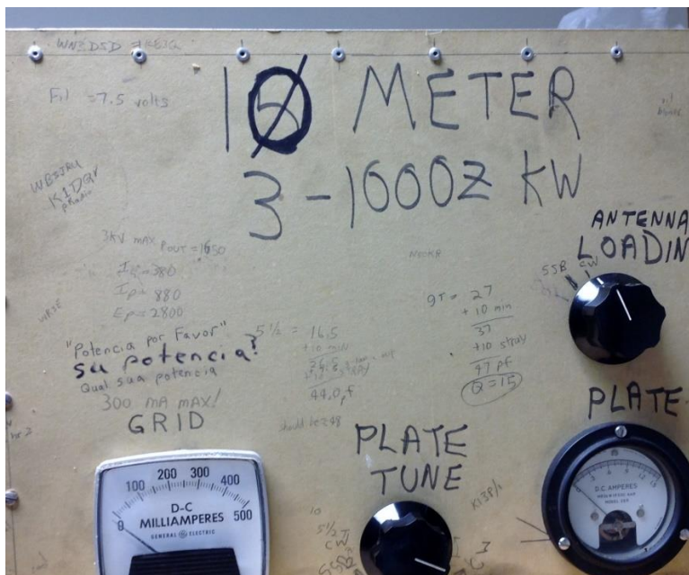
The 10 meter amp at W3LPL, showing state of the art front panel labeling techniques...
